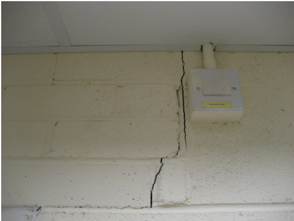
27. Example of internal cracking
