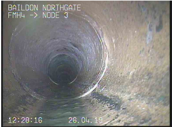
FMH4X_856a3b63-4c27-4a91-95e7-18b0a7d1567e_20190426_132821_789.jpg, 00:04:14, 14.45m Crack, circumferential at joint from 12 o'clock to 12 o'clock
