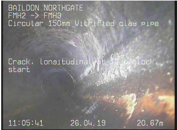
FMH2X_dfac9445-7789-42f9-9c93-5412efc5cae5_20190426_120545_917.jpg, 00:06:37, 20.67m Crack, longitudinal at 12 o'clock, start
