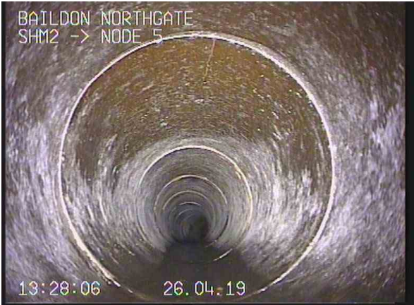
SHM2X_b39c3297-7e97-4427-a986-ace9cd0ff24_20190426_142811_657.jpg, 00:00:33, 1.97m Crack, longitudinal at joint at 12 o'clock
