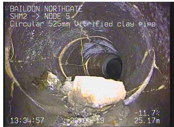
SHM2X_2c0e3a17-0613-405e-b321-cad5f463677d_20190426_143502_372.jpg, 00:05:32, 25.17m Cracks, multiple from 12 o'clock to 12 o'clock, finish
