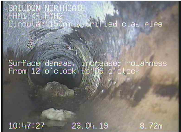
FHM1X_da6e11aa-340a-490b-9029-361575704d35_20190426_114731_845.jpg, 00:02:17, 8.72m Surface damage, increased roughness from 12 o'clock to 06 o'clock
