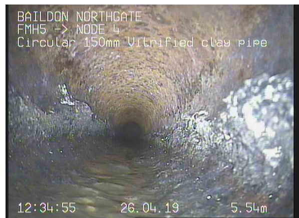
FMH5X_481421fb-d2cb-4509-8f93-f3d2439639d6_20190426_133500_046.jpg, 00:01:54, 5.54m Attached deposits, grease from 03 o'clock to 09 o'clock, 10% cross-sectional area loss
