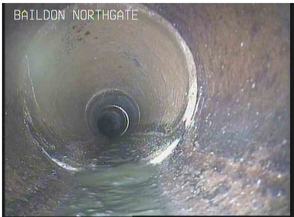
FMH4X_b5e1c4cf-d5b9-4ecb-b6c5-60dc9ea2eb7d_20190426_132538_882.jpg, 00:02:33, 10.44m Cracks, multiple at joint from 06 o'clock to 01 o'clock
