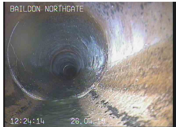
FMH4X_d089155c-a662-418a-8793-6fc2c406b2af_20190426_132419_552.jpg, 00:01:47, 7.30m Cracks, multiple at joint from 07 o'clock to 10 o'clock
