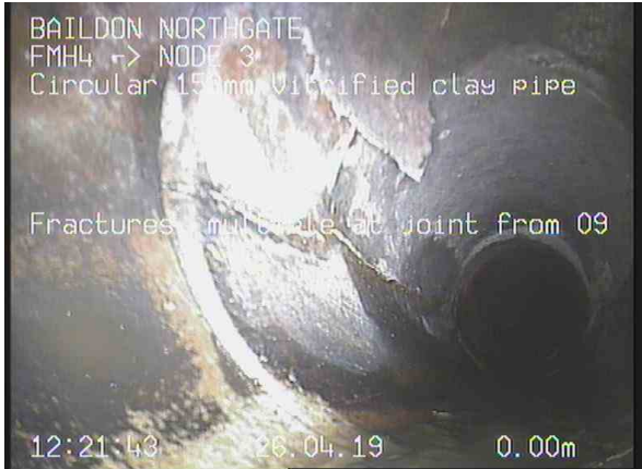
FMH4X_b51d49de-b6f7-40d0-9670-62a95d0827c4_20190426_132148_197.jpg, 00:00:12, 0.10m Fractures, multiple at joint from 09 o'clock to 12 o'clock
