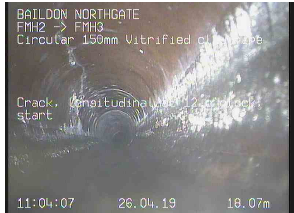
FMH2X_9bb14d8b-ff7f-440a-94cd-94cb75ddfedf_20190426_120412_187.jpg, 00:05:36, 18.07m Crack, longitudinal at 12 o'clock, start
