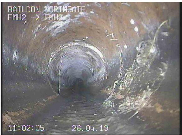
FMH2X_3a386f54-5308-447b-b41d-55cf66ec0d0f_20190426_120210_609.jpg, 00:04:02, 13.92m Cracks, multiple from 12 o'clock to 06 o'clock
