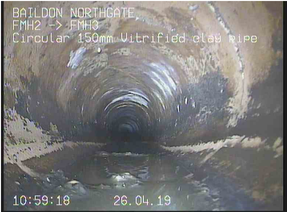
FMH2X_e441ac73-54a0-4fd0-aa70-d03f2ddc3234_20190426_115923_522.jpg, 00:01:51, 4.23m Fractures, multiple from 12 o'clock to 12 o'clock
