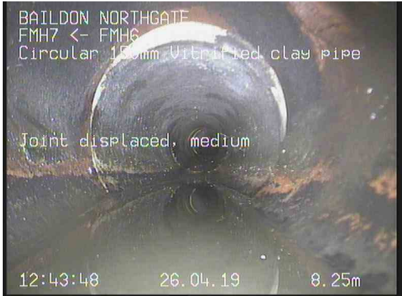
FMH7X_773b61af-2212-40eb-8553-b481a60c6293_20190426_134353_603.jpg, 00:01:36, 8.25m Joint displaced, medium
