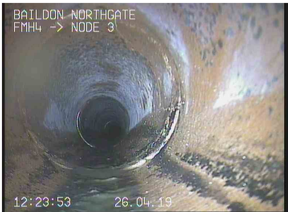
FMH4X_8f6b01eb-ef32-444e-8954-16e455c3c3d2_20190426_132358_283.jpg, 00:01:36, 6.74m Cracks, multiple at joint from 12 o'clock to 12 o'clock
