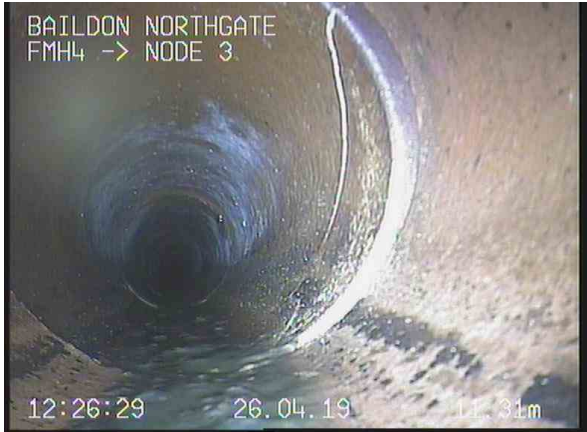
FMH4X_078ea355-74d4-4c82-aa47-65076ffb2622_20190426_132634_287.jpg, 00:03:03, 11.31m Fracture, circumferential at joint from 01 o'clock to 06 o'clock
