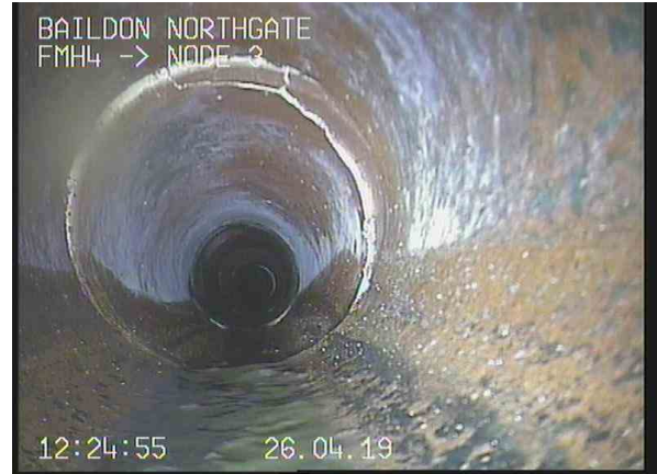
FMH4X_572d9478-faec-4a76-a82a-f8f6e0bfd02f_20190426_132500_617.jpg, 00:02:11, 9.11m Cracks, multiple at joint from 11 o'clock to 04 o'clock
