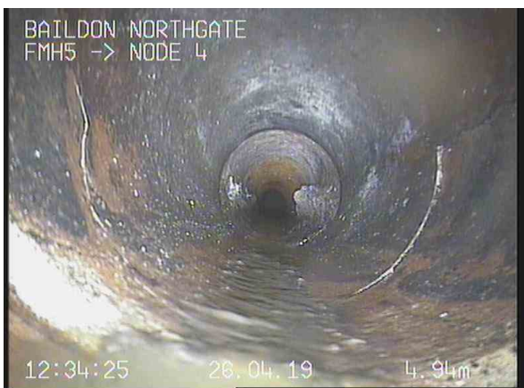
FMH5X_05e85977-87fd-4c18-97dc-d1236d17314d_20190426_133430_527.jpg, 00:01:41, 4.94m Fractures, multiple from 03 o'clock to 09 o'clock
