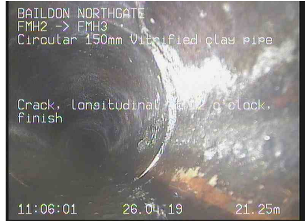
FMH2X_9ed07a0f-87b0-44cc-8256-ec9a3b873836_20190426_120606_383.jpg, 00:06:52, 21.25m Crack, longitudinal at 12 o'clock, finish
