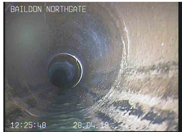
FMH4X_37f6b874-9d80-4475-bc17-4a5e625a9776_20190426_132553_689.jpg, 00:02:42, 10.67m Crack, longitudinal at joint at 12 o'clock
