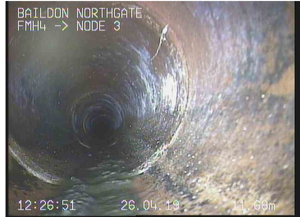
FMH4X_7ddf25d9-c04a-46e7-88d6-8f996d0a5c22_20190426_132656_057.jpg, 00:03:16, 11.68m Crack, longitudinal at joint at 02 o'clock
