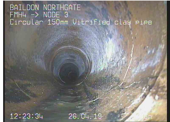
FMH4X_4481a01b-925b-4542-8f02-356f730d7c44_20190426_132339_203.jpg, 00:01:23, 5.86m Fractures, multiple from 12 o'clock to 12 o'clock
