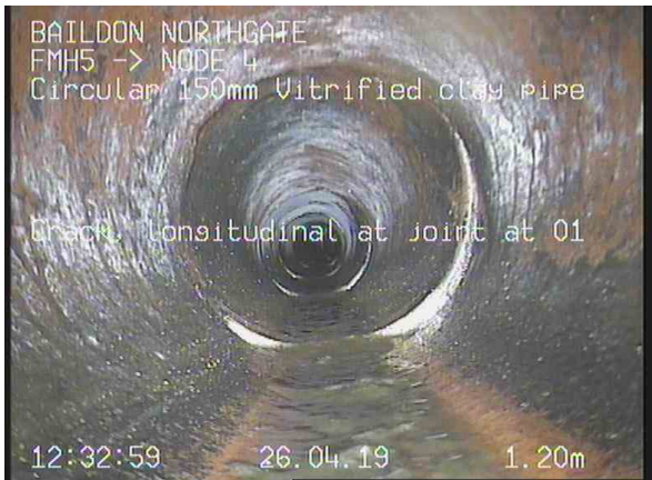
FMH5X_6d62e0e6-e35b-4c66-8896-8f3e35199cab_20190426_133304_557.jpg, 00:00:37, 1.19m Crack, longitudinal at joint at 01 o'clock
