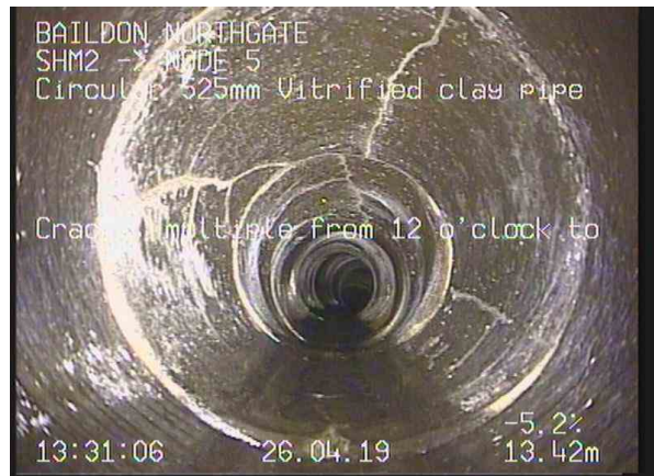
SHM2X_76e72302-4cb0-4400-ac83-4a4521799b0b_20190426_143111_219.jpg, 00:02:40, 13.42m Cracks, multiple from 12 o'clock to 12 o'clock, start
