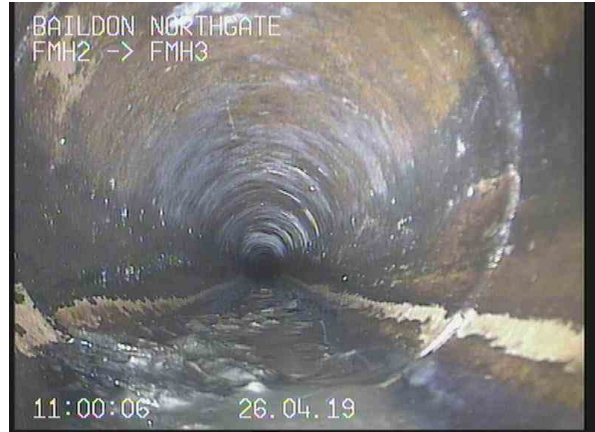
FMH2X_fed6c56c-b69e-404e-a153-260b08a9bd37_20190426_120011_601.jpg, 00:02:19, 5.02m Crack, longitudinal at 12 o'clock
