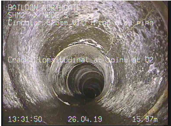
SHM2X_60a6810e-aed7-482a-b788-89612660317b_20190426_143155_865.jpg, 00:03:13, 15.97m Crack, longitudinal at joint at 02 o'clock
