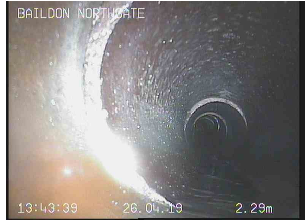
NODE 6X_e776eb2f-4ddb-4987-af8b-8e59e9d2e7ac_20190426_144 344_749.jpg, 00:00:50, 2.29m Joint displaced, medium
