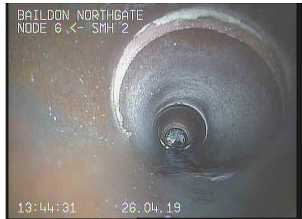
NODE 6X_ea13d6de-62ea-4f21-a3c1-8d536d0f3a64_20190426_144 436_539.jpg, 00:01:26, 4.65m Joint displaced, medium
