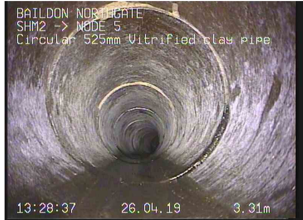
SHM2X_74e081c4-76cd-4b14-bffb-17f9eee899d6_20190426_142842_223.jpg, 00:00:54, 3.31m Crack, longitudinal at 12 o'clock
