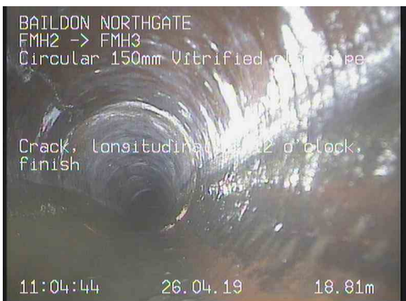
FMH2X_071e6193-0d9f-4261-ba4c-99cdd0e711f2_20190426_120449_518.jpg, 00:06:00, 18.81m Crack, longitudinal at 12 o'clock, finish
