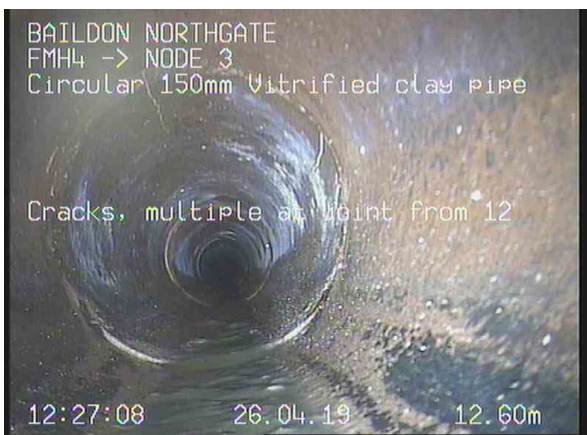
FMH4X_37a5d84a-854c-404b-a321-1172a2489fd6_20190426_132713_349.jpg, 00:03:26, 12.60m Cracks, multiple at joint from 12 o'clock to 12 o'clock
