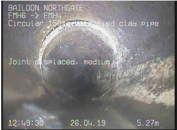
FMH6X_73c610c7-1ed0-4ca8-bae9-efec823b5e9a_20190426 _134935_867.jpg, 00:00:59, 5.27m Joint displaced, medium
