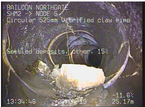
SHM2X_e59c87d4-d43d-4762-8906-aa34cd9aa7a8_20190426_143451_842.jpg, 00:05:27, 25.17m Settled deposits, other, 15% cross-sectional area loss
