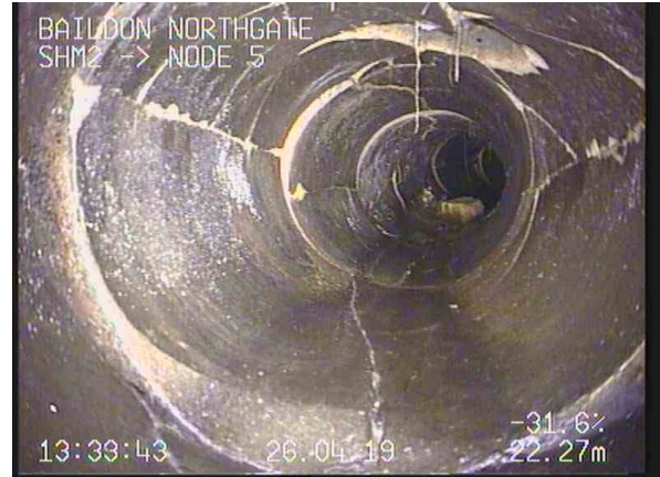
SHM2X_6cbad2c2-0f0c-41bb-9652-0fb188b4c837_20190426_143348_461.jpg, 00:04:48, 22.24m Hole in drain or sewer from 11 o'clock to 01 o'clock
