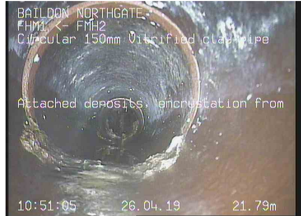
FHM1X_e696a407-eba3-42f9-9374-6ce6d4706b81_20190426_115110_459.jpg, 00:04:57, 21.79m Attached deposits, encrustation from 05 o'clock to 08 o'clock, 5% cross-sectional area loss
