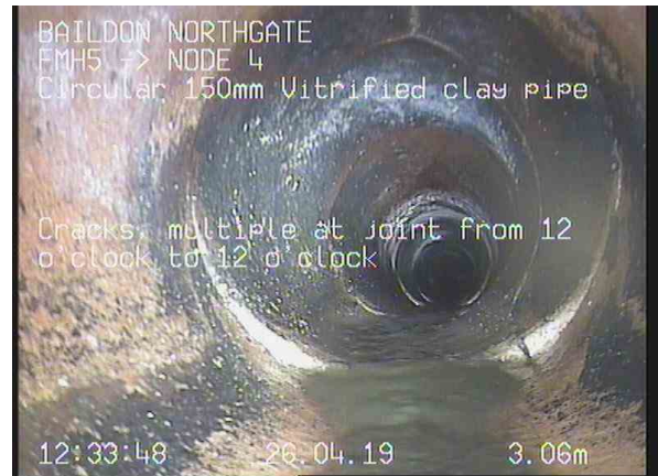
FMH5X_8c712ea2-c648-4554-b87e-865940ebdf75_20190426_133353_669.jpg, 00:01:13, 3.06m Cracks, multiple at joint from 12 o'clock to 12 o'clock
