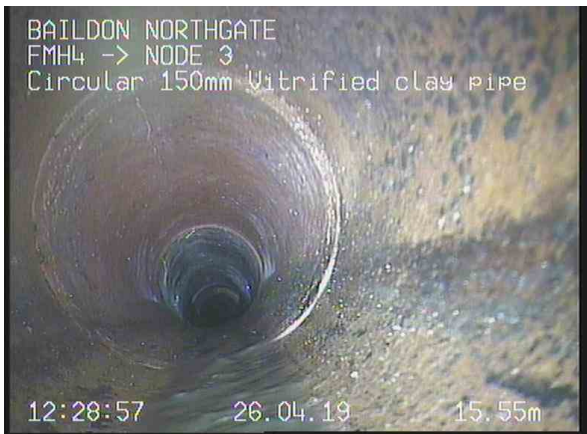
FMH4X_5c6cca82-9a4d-47a1-baeb-070ccae904a1_20190426_132902_294.jpg, 00:04:41, 15.55m Crack, longitudinal at joint at 12 o'clock
