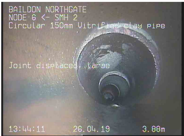
NODE 6X_433d8569-b191-460b-9036-0d176aa812a9_20190426_14 4416_603.jpg, 00:01:08, 3.88m Joint displaced, large
