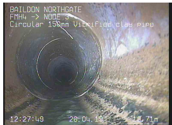
FMH4X_836c0e56-3f37-43fa-bdf4-4936ccdd71c1_20190426_132754_154.jpg, 00:03:55, 13.71m Fractures, multiple at joint from 12 o'clock to 12 o'clock
