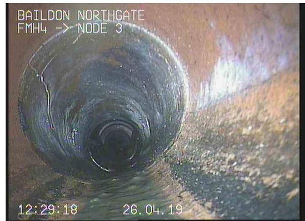
FMH4X_f9ab6ddc-9c77-48c3-b4e5-4af9b806b68f_20190426_132923_052.jpg, 00:04:53, 16.09m Fractures, multiple at joint from 06 o'clock to 12 o'clock
