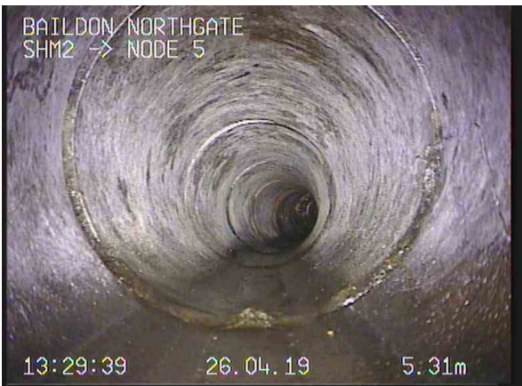
SHM2X_bdb853b0-9749-4c59-b2c0-6666ebbc300d_20190426_142945_169.jpg, 00:01:28, 5.31m Crack, circumferential at joint from 03 o'clock to 05 o'clock
