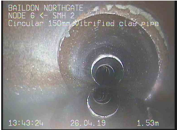
NODE 6X_9da08712-1f0e-4fee-91a5-18e7db945014_20190426_144 329_343.jpg, 00:00:38, 1.53m Joint displaced, large
