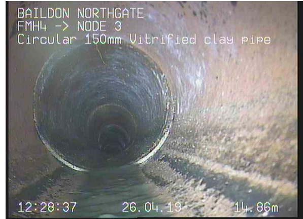
FMH4X_94a441cb-1ccb-48af-b4db-29b1968e9864_20190426_132842_470.jpg, 00:04:27, 14.86m Crack, longitudinal at joint at 12 o'clock
