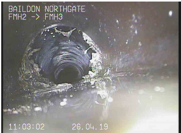
FMH2X_5ccfeccc-0854-4eea-b5c7-b669a8242c0c_20190426_120307_092.jpg, 00:04:46, 16.73m Roots, mass, 10% cross-sectional area loss
