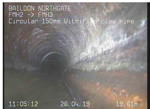
FMH2X_ef0ce60b-3d71-431e-92f8-2f758fc0a796_20190426_120517_313.jpg, 00:06:17, 19.61m Crack, longitudinal at 12 o'clock
